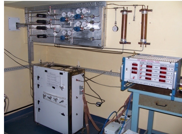
4 gas mixing unit
